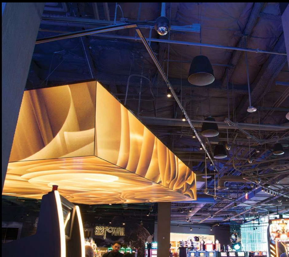
Ten 12-inch pendant speakers surround this central bar in the main casino.
